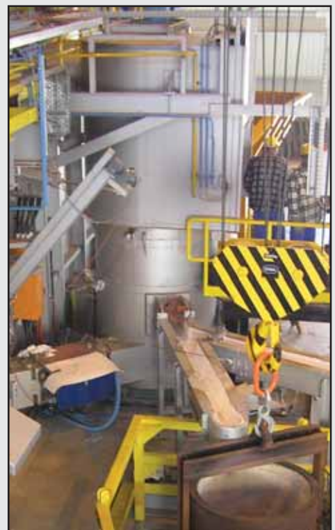
Recently installed EMP system operating in customer's plant
