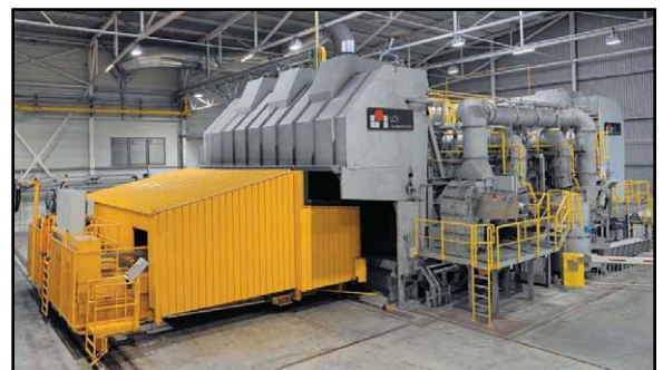
LOI 50,000 mt/yr twin-chamber furnace installed in 2009 as part of Hydro/Novelis' new recycling centre at Alunorf, Neuss, Germany
